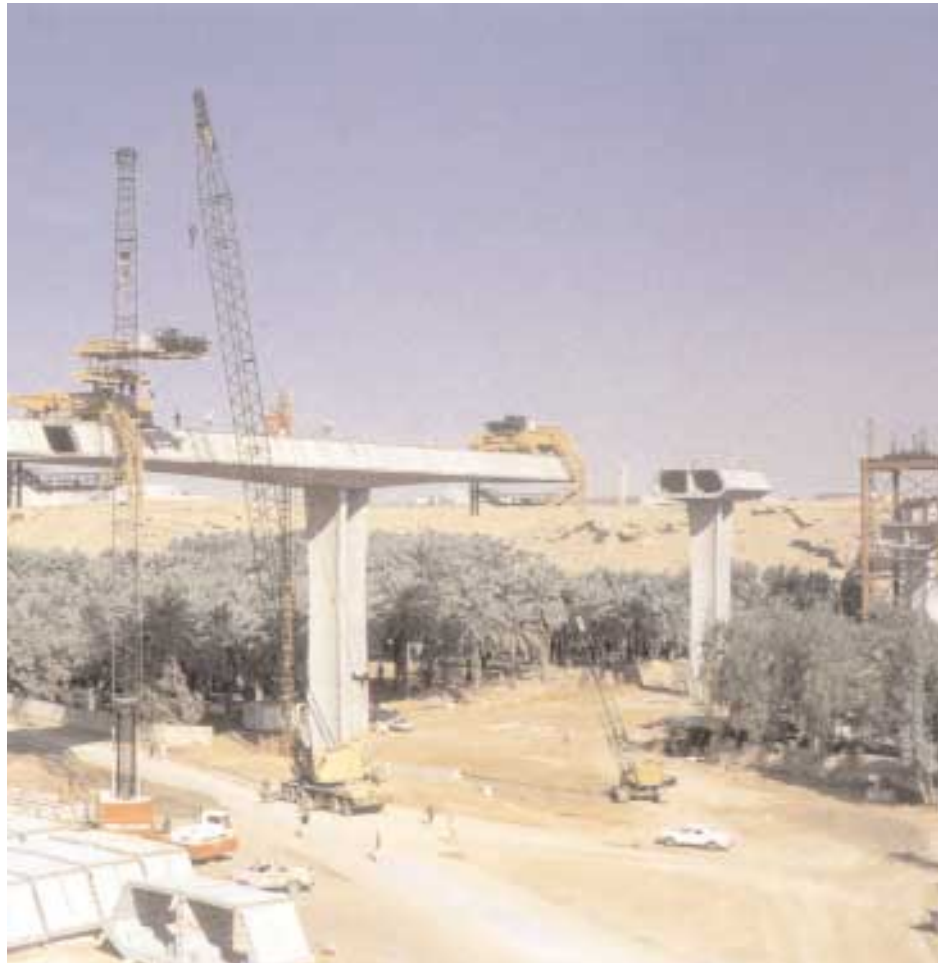
VSL work included lifting and placement of pier heads, spine segments and side frames, as well as longitudinal and transverse post-tensioning of the superstructure.
