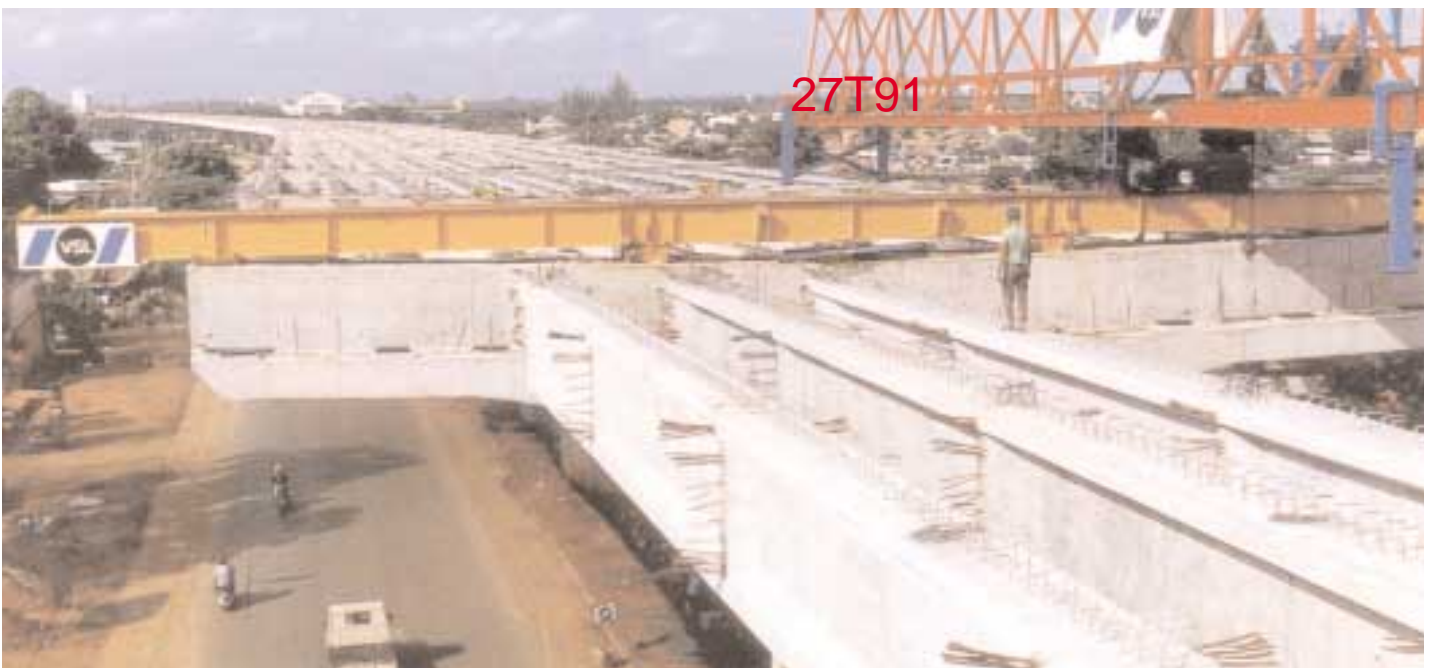
VSL Launching Gantry placed a total of 4,100 I-beams, averaging 200 beams per month.
