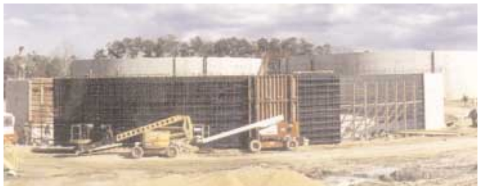
Clarifier tank was designed with corrosion protected CP + monostrand tendons in vertical and horizontal directions.
